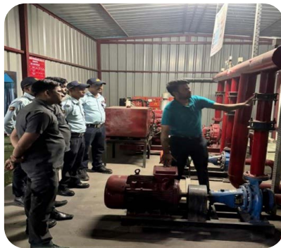
Fire pump room training
